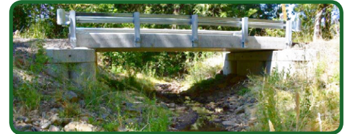
Top: Culvert blocks salmon trying to get home. Bottom: Bridge allows salmon to swim through.
